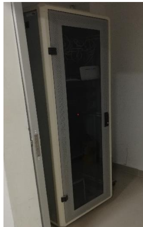
INTERIOR DATA CENTER
